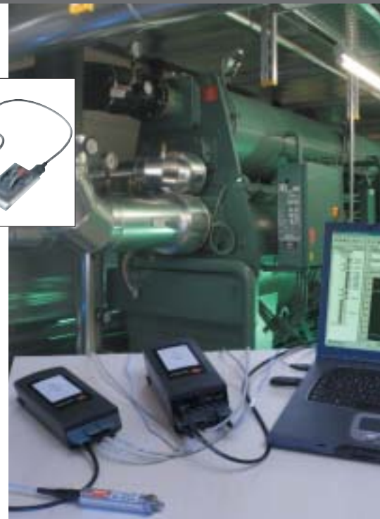
Measure superheating/subcooling and the oil pressure in an industrial refrigeration system
