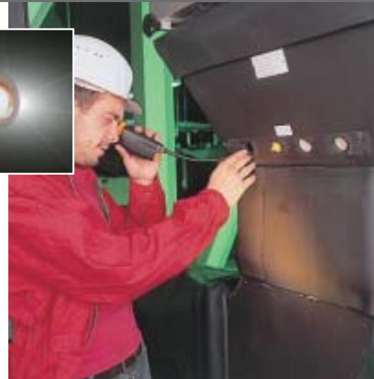
Easy detection of blocked air conditioning ducts
