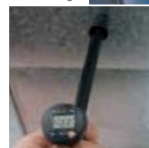
Measurement in VAC duct with duct holder
